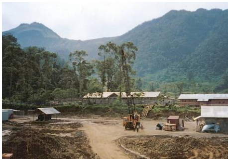
Work camp for construction of 52 MW Mindanao I in 1996. Mt. Apo, the highest point in the Philippines, can be seen in the background to the left.
