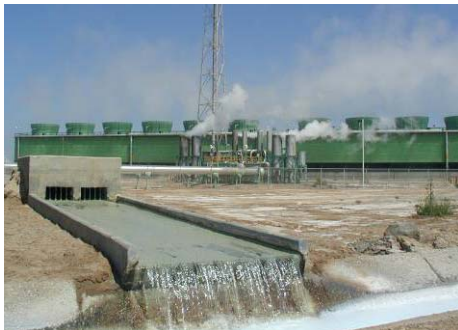
100 MW Cerro Prieto IV, Mexico – 2001.
