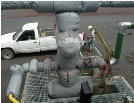
The new wellhead at Puna, 2003.
