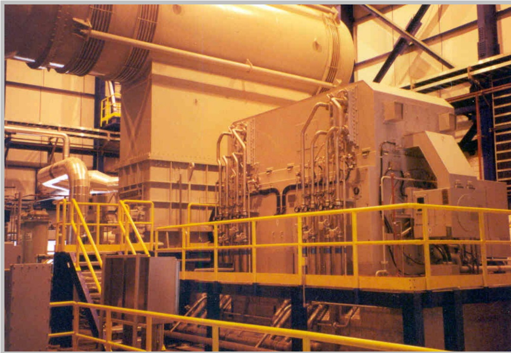
The tall structure in the background is the turbine housing and steam exhaust duct; the boxy component at the right is the electrical generator.
