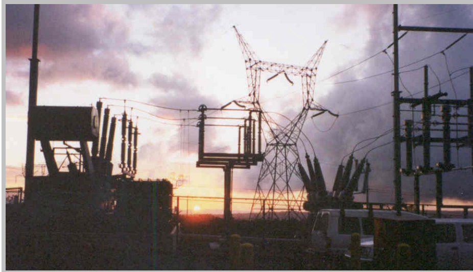
A view from the Miravalles III 230kV substation.
