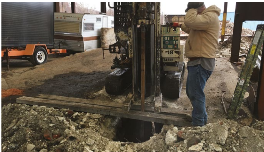
Drilling time. A track-mounted GeoProbe rig is used to conduct Phase II soil sampling at a former foundry. Over three feet of historic, layered concrete floors are excavated before sampling of subsurface soils can begin.
