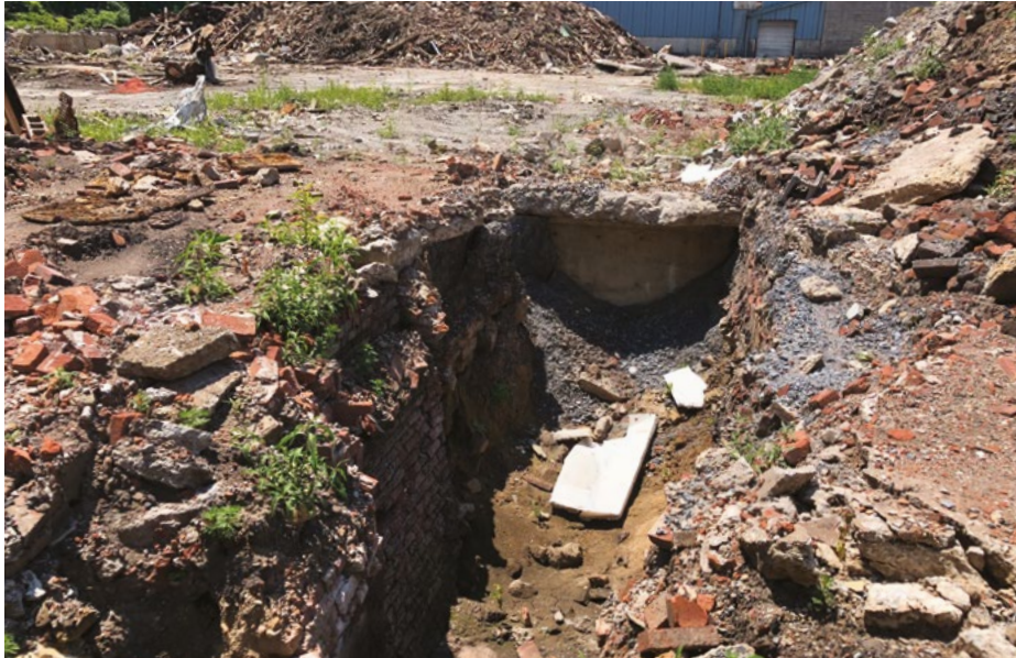
Soil investigation. A three-foot trench is dug to conduct Phase II soil sampling for metals and other contaminants adjacent to former building foundations.
